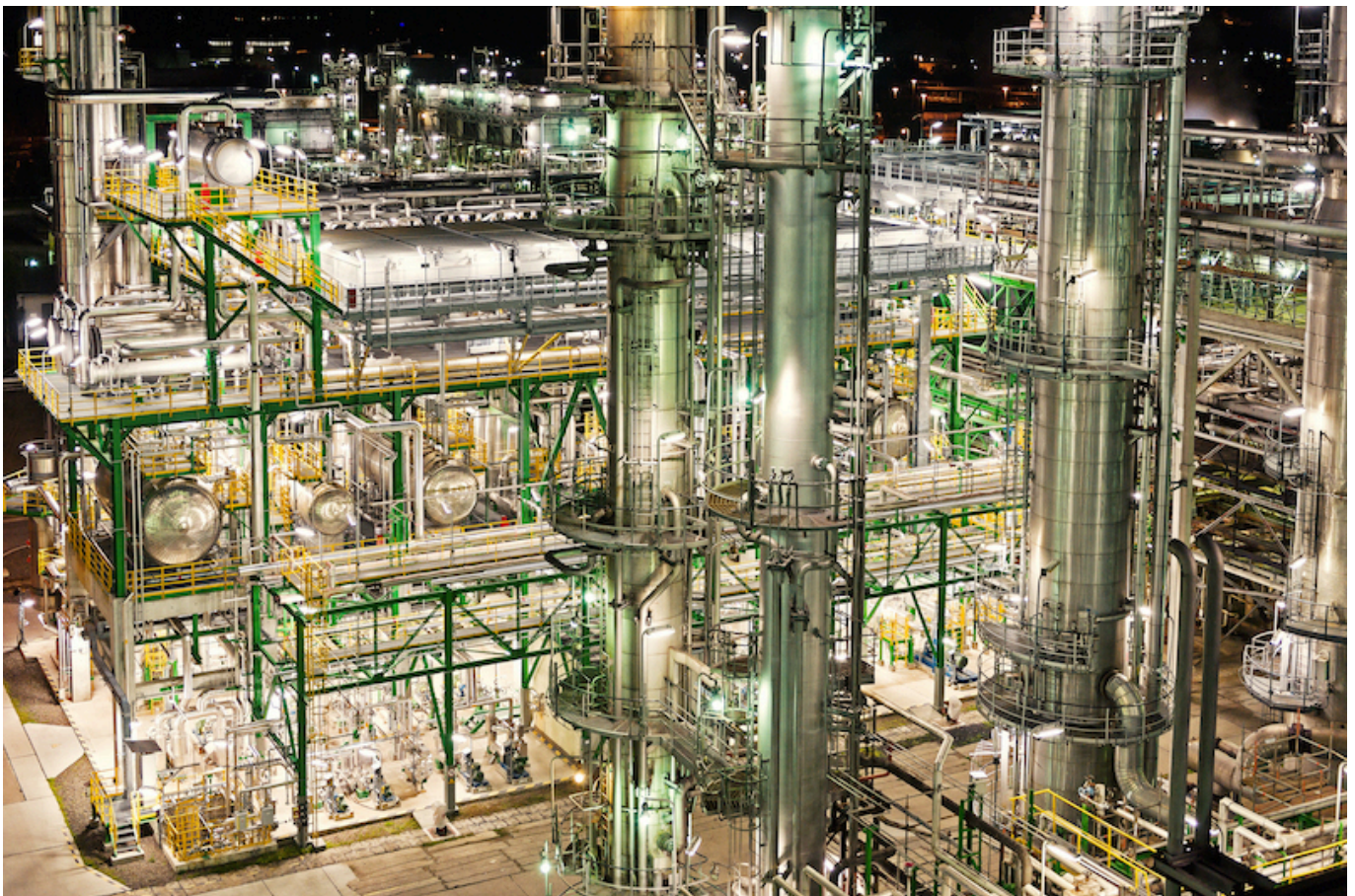
Copyright PCK Raffinerie GmbH
